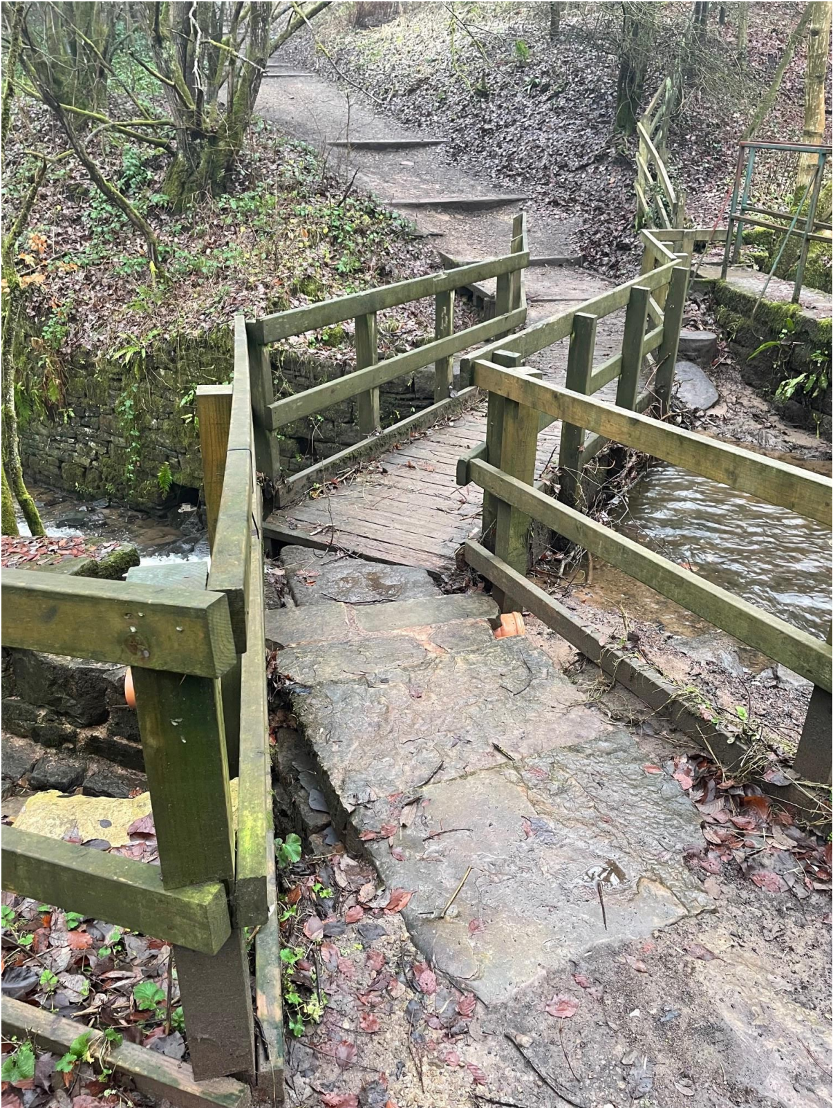
Photograph 1: Shows the access onto Footpath 26 from the informal footpath from Ashbrook Road
